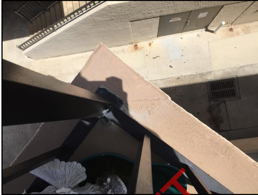
Photograph 41: Unit #401, Leading edge of balcony cracked and spalling.
