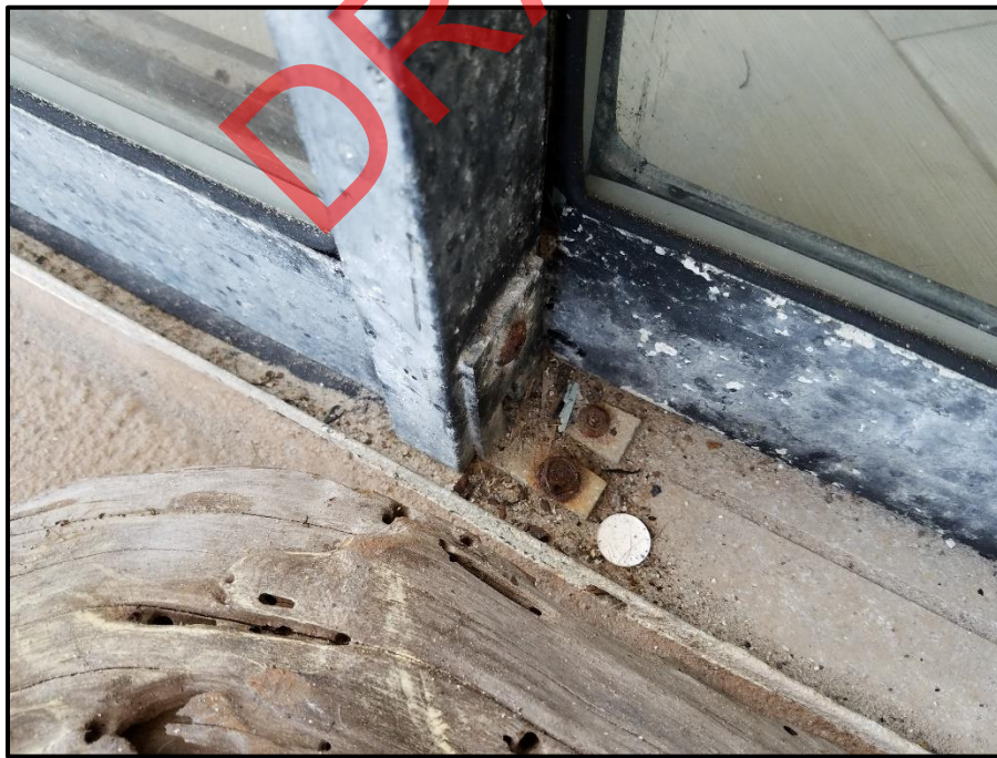
Photograph 76: Unit #303, Sliding glass door fasteners heavily corroded.
