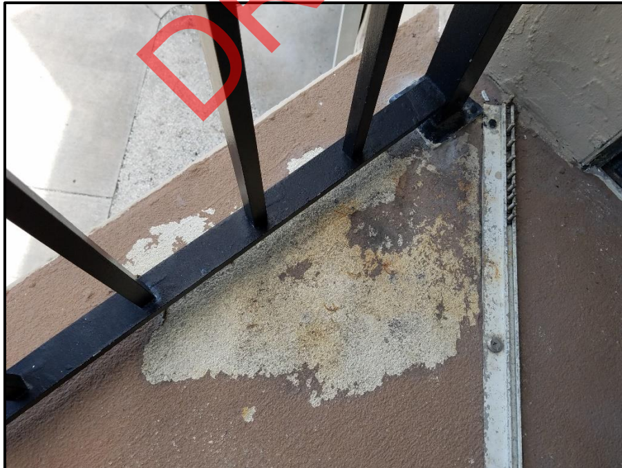
Photograph 78: Unit #303, Acrylic coating failure observed.
