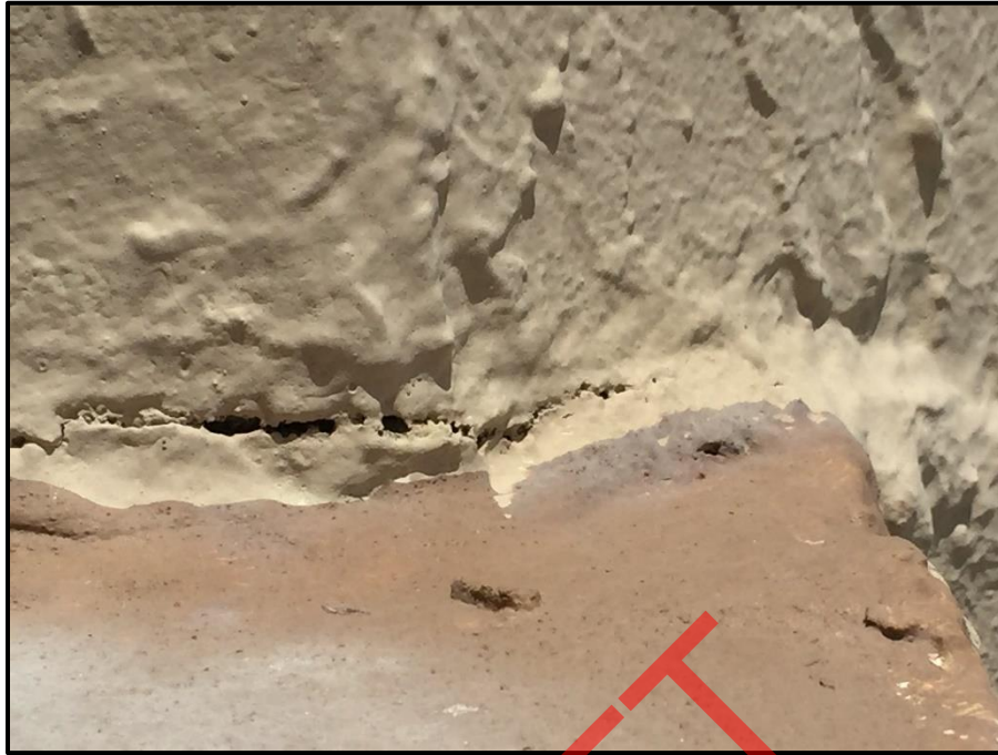
Photograph 49: Unit #404, Sealant failure at unit wall.
