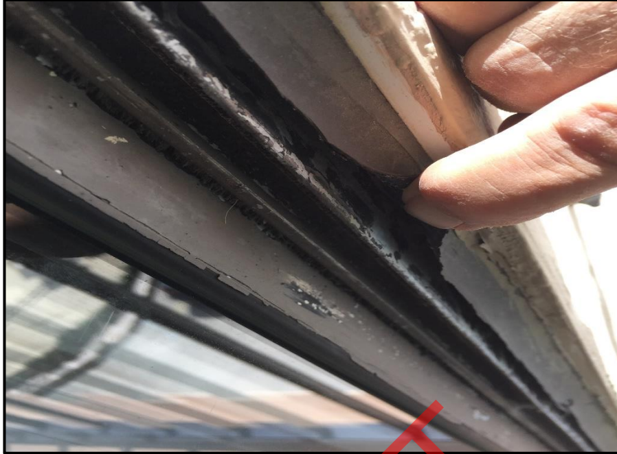
Photograph 39: Unit #403, Sliding glass door sealant failure.
