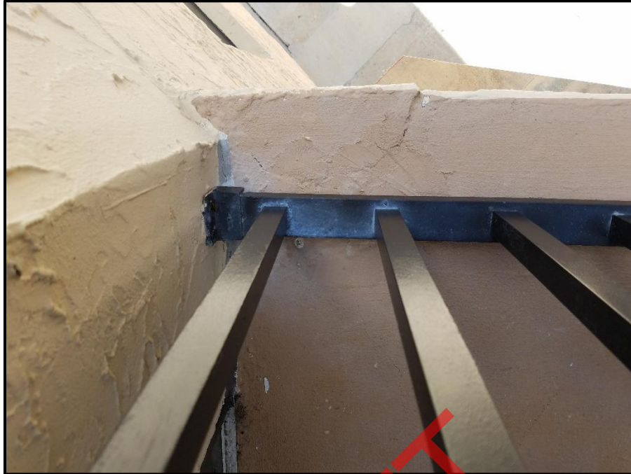
Photograph 65: Unit #301, Balcony cracked and spalling at leading edge and unit wall.
