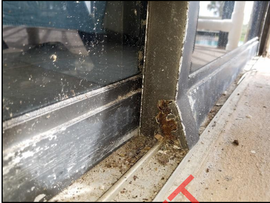
Photograph 11: Unit #203, Sliding glass doors heavily corroded due to long term salt exposure.
