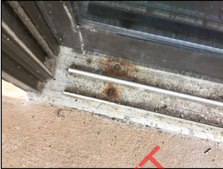
Photograph 61: Unit #202, Sliding glass door fasteners heavily corroded and potential source of water intrusion.
