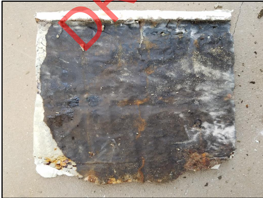
Photograph 68: Unit #301, Felt paper at back side of stucco sample stained with rust due to long term water intrusion.
