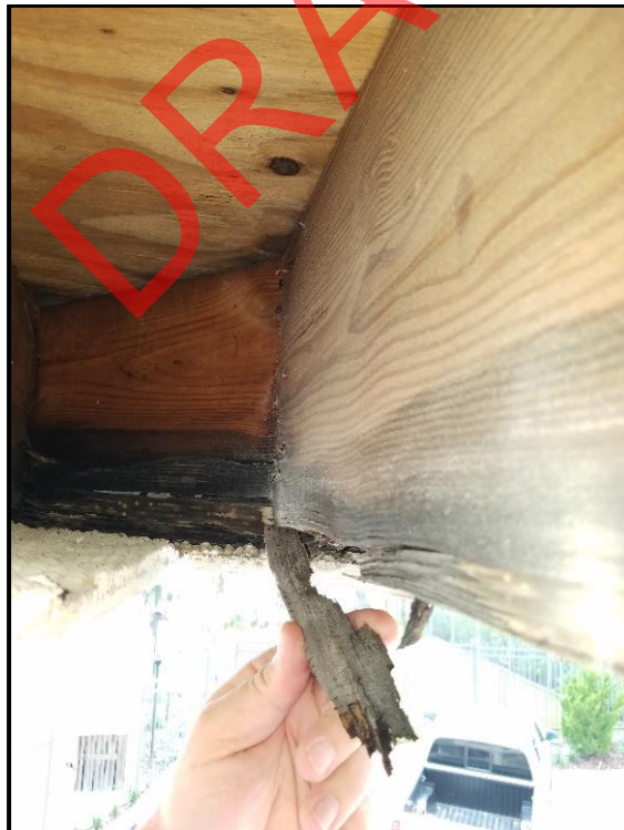
Photograph 4: Unit #203, Bottom edge of floor joist severely rotted.
