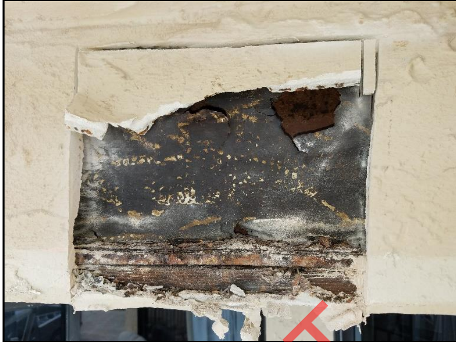
Photograph 5: Unit #203, Observation hole cut in stucco at structural I-beam. Felt paper stained due to water intrusion.
