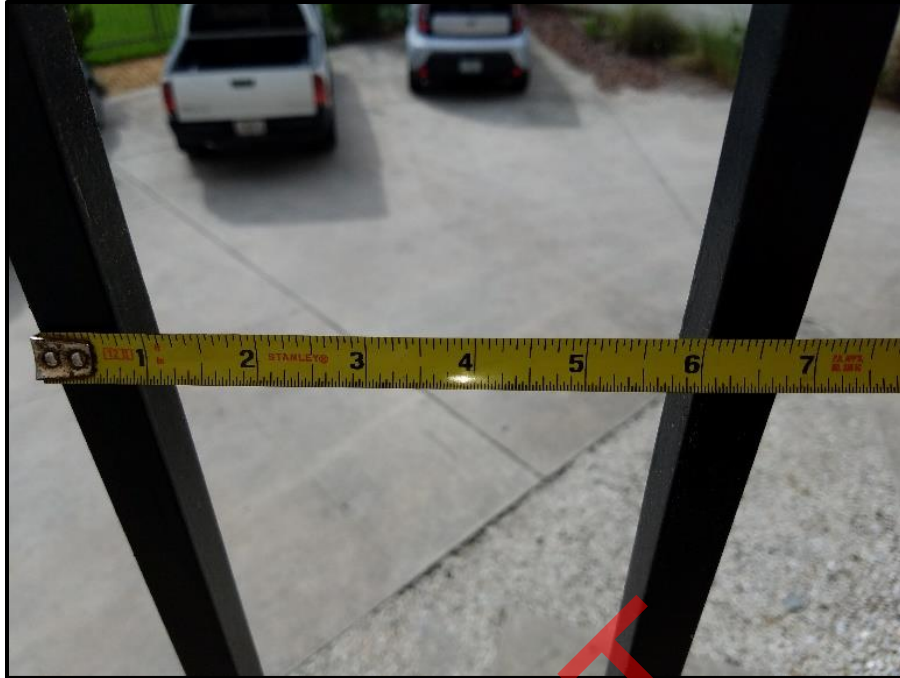
Photograph 9: Unit #203, Guardrail picket spacing exceeds code requirement of less than 4 inches.
