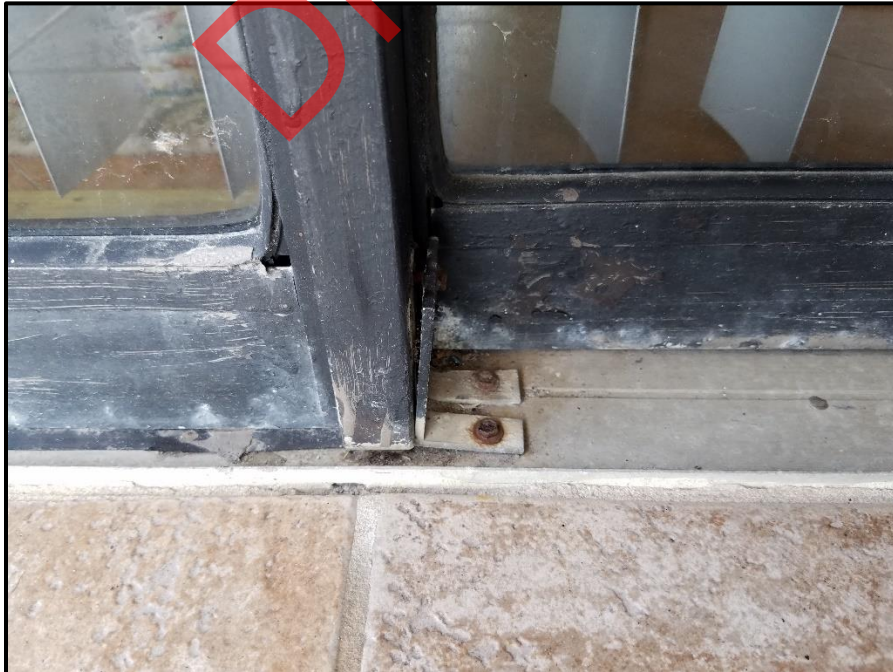
Photograph 32: Unit #402, Corroded fasteners observed at sliding glass door threshold.
