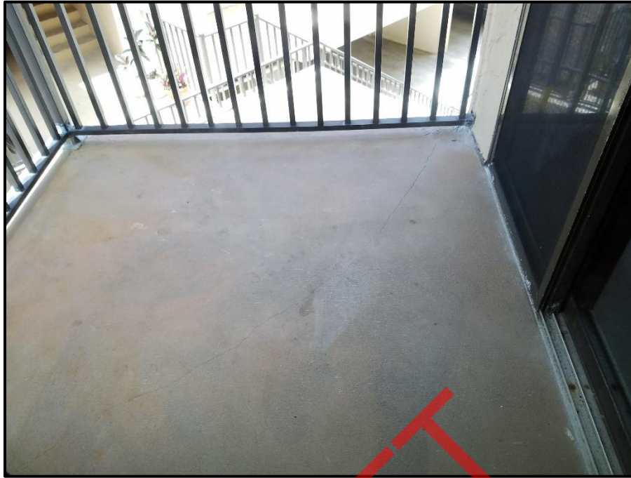
Photograph 63: Unit #301, Balcony topping slab cracked down the middle.
