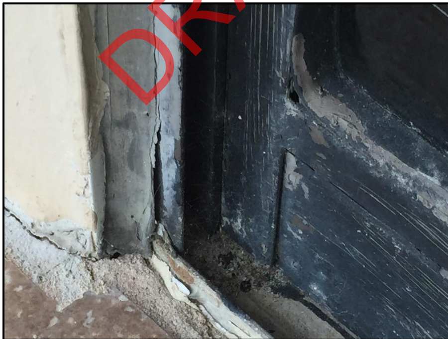
Photograph 34: Unit #402, Sealant failure at sliding glass door and unit wall.
