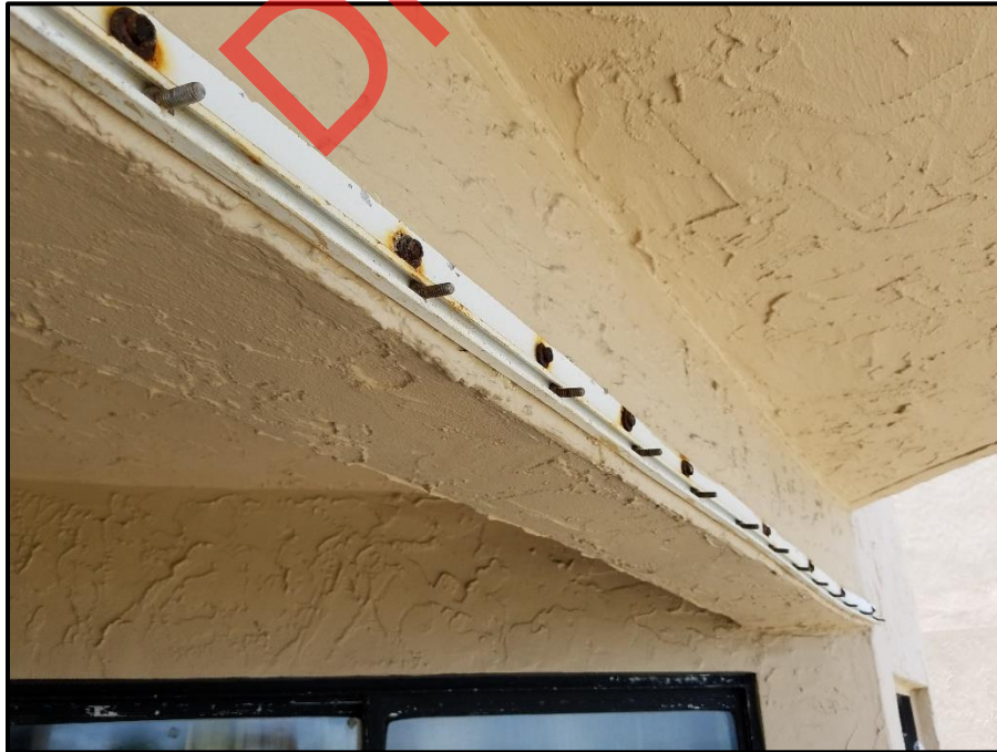
Photograph 80: Unit #303, Storm shutter fasteners heavily corroded and potential source of water intrusion.
