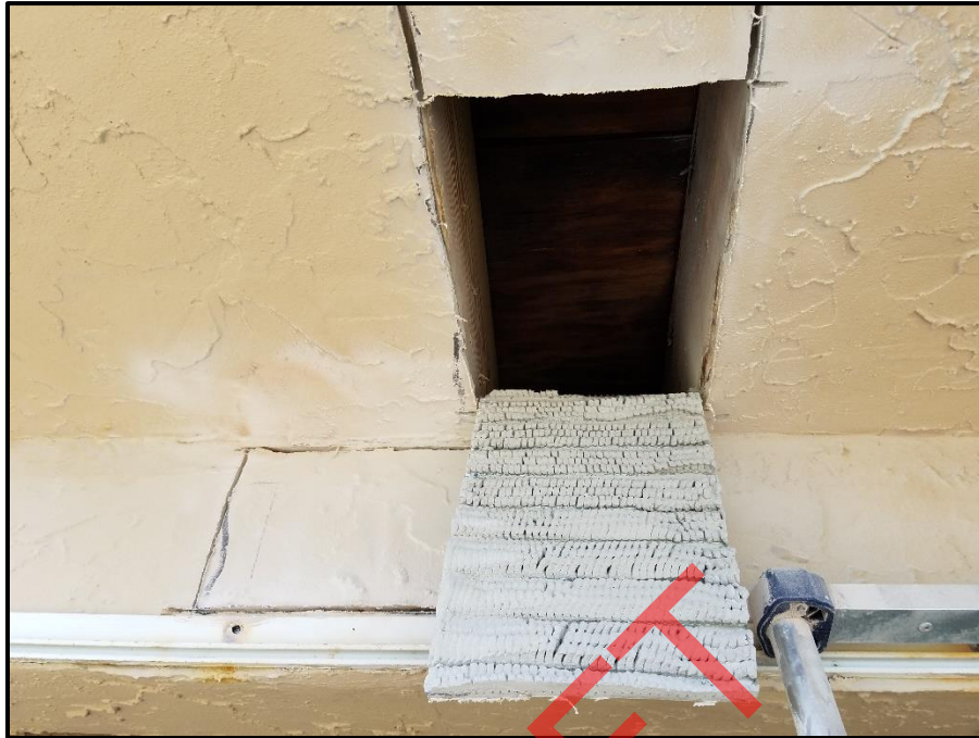
Photograph 81: Unit #304, Observation hole cut at ceiling and I-beam location.
