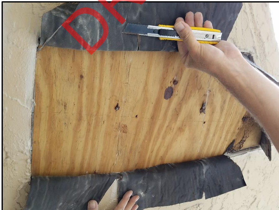
Photograph 16: Unit #204, new(er) plywood sheathing at balcony ceiling.
