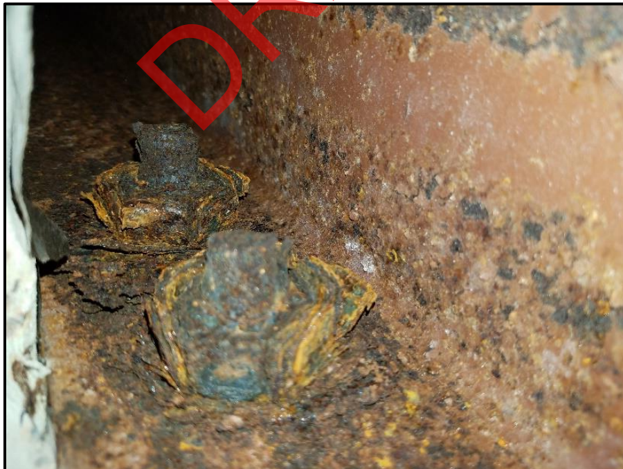
Photograph 8: Unit #203, I-beam fasteners severely corroded due to long term water intrusion.
