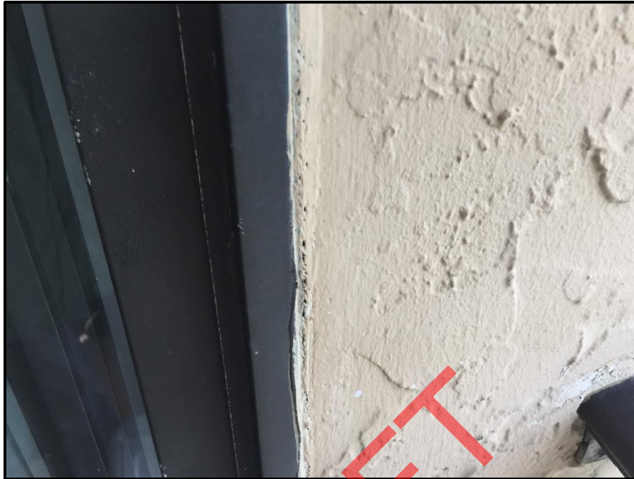
Photograph 51: Unit #404, Sealant failure at sliding glass door.
