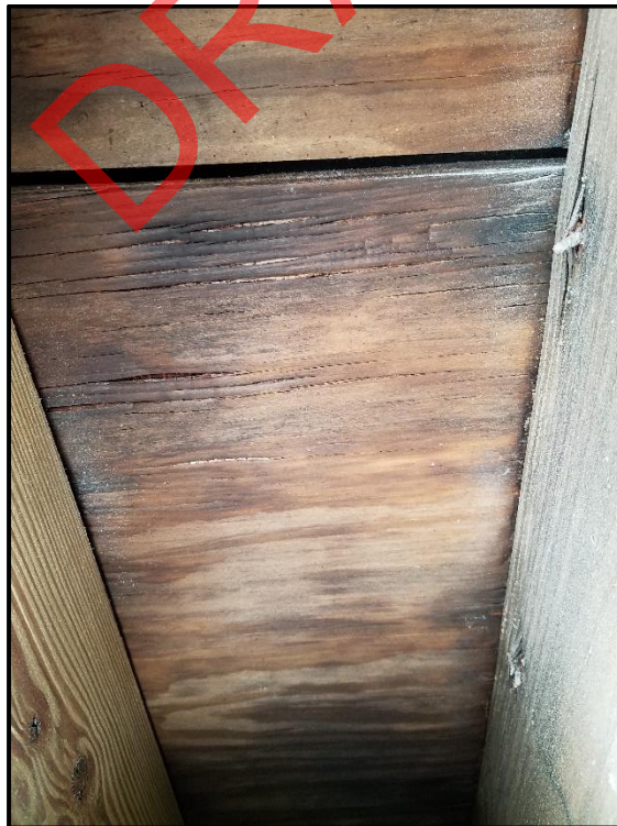
Photograph 82: Unit #304, Underside of deck sheathing stained and saturated due to water intrusion.
