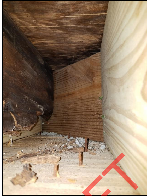
Photograph 19: Unit #204, Interior view of ceiling cavity. Decayed decking.
