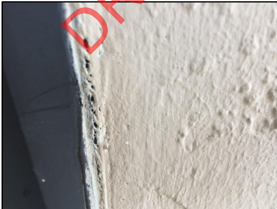
Photograph 52: Unit #404, Close of previous photo.
