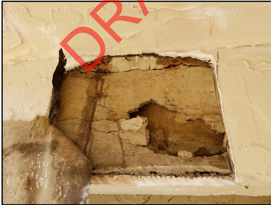
Photograph 58: Unit #202, Same location as previous photo.
