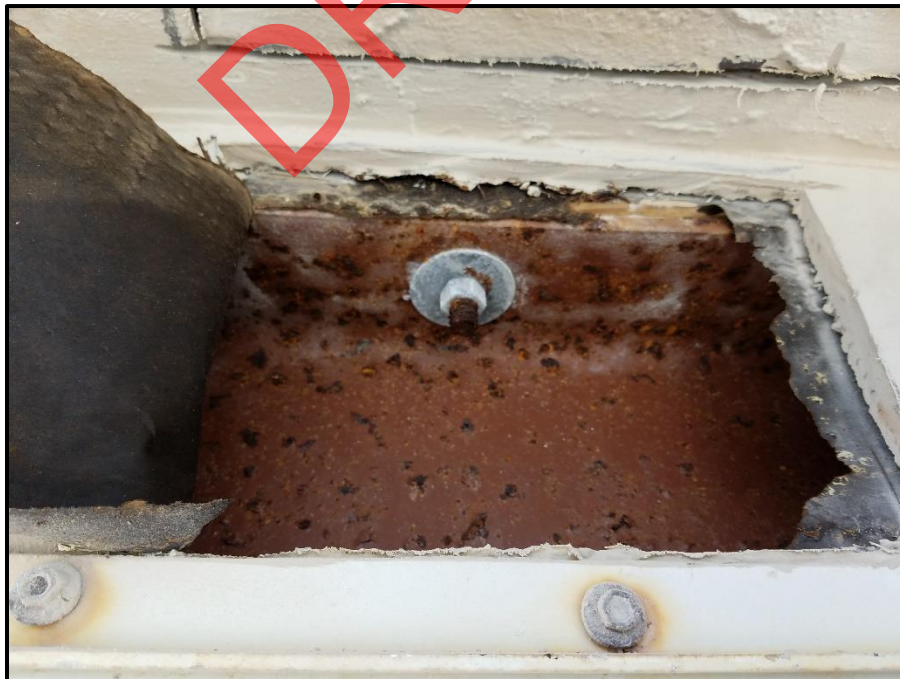
Photograph 74: Unit #303, I-beam and fasteners beginning to corrode.
