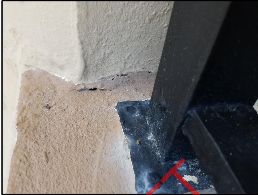
Photograph 79: Unit #303, Sealant failure at unit wall.
