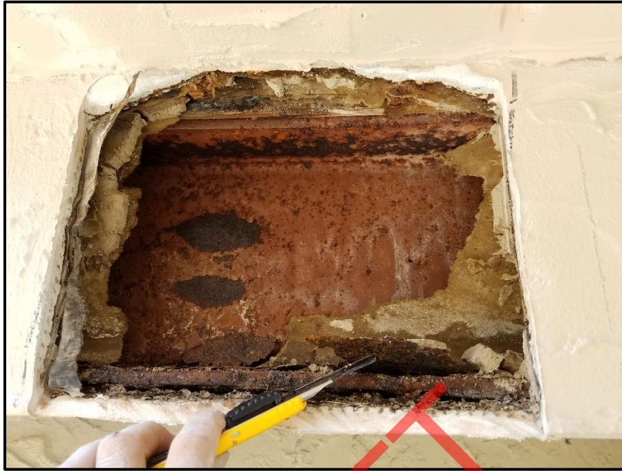
Photograph 69: Unit #301, I-beam corrosion observed.
