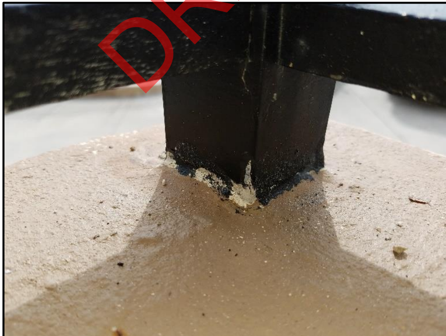
Photograph 10: Unit #203, Guardrail post corrosion (aluminum oxide).
