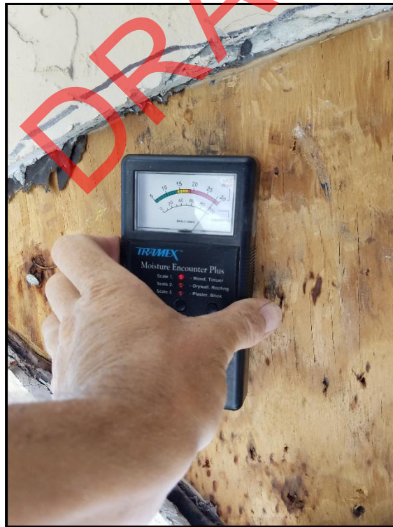
Photograph 54: Unit #202, Readings taken indicate high level of moisture contained in plywood sheathing.
