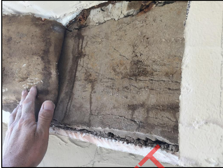
Photograph 57: Unit #202, Gyp board installed upon original construction saturated due to long term water intrusion.
