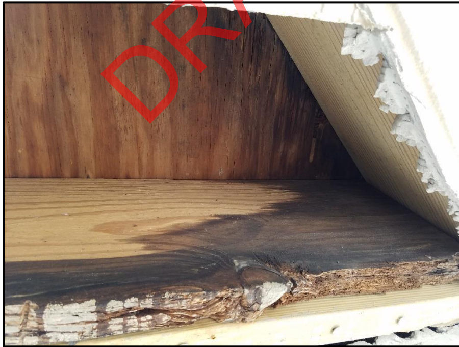
Photograph 72: Unit #303, New joist attached to old joist indicating previous repair attempt.
