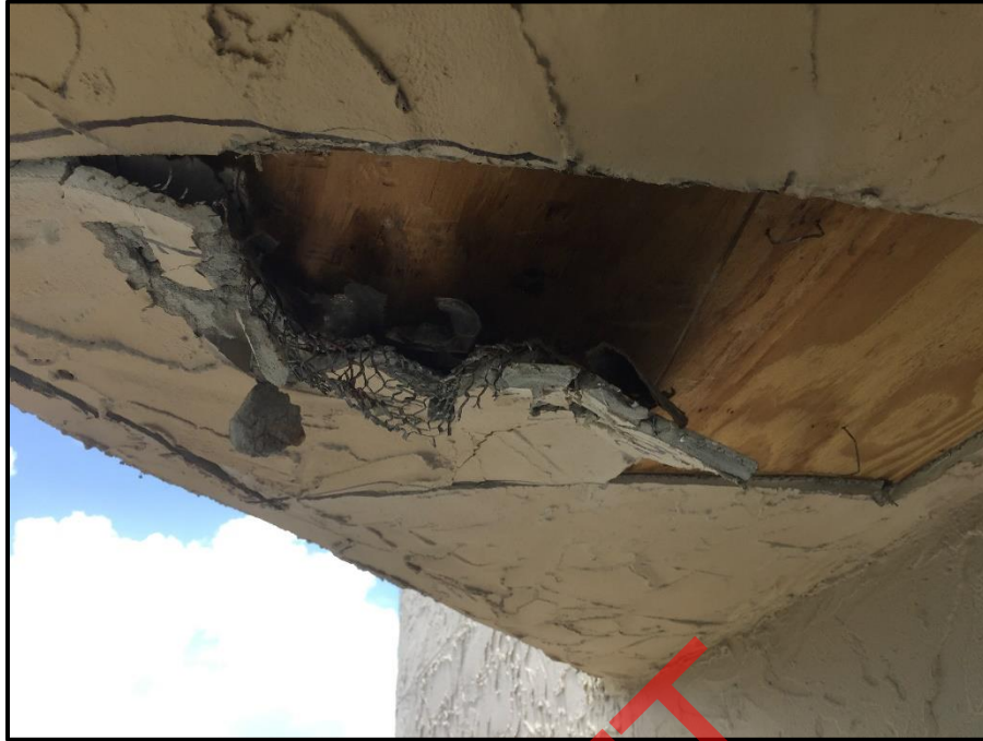
Photograph 53: Unit #202, Observation hole cut in stucco ceiling.
