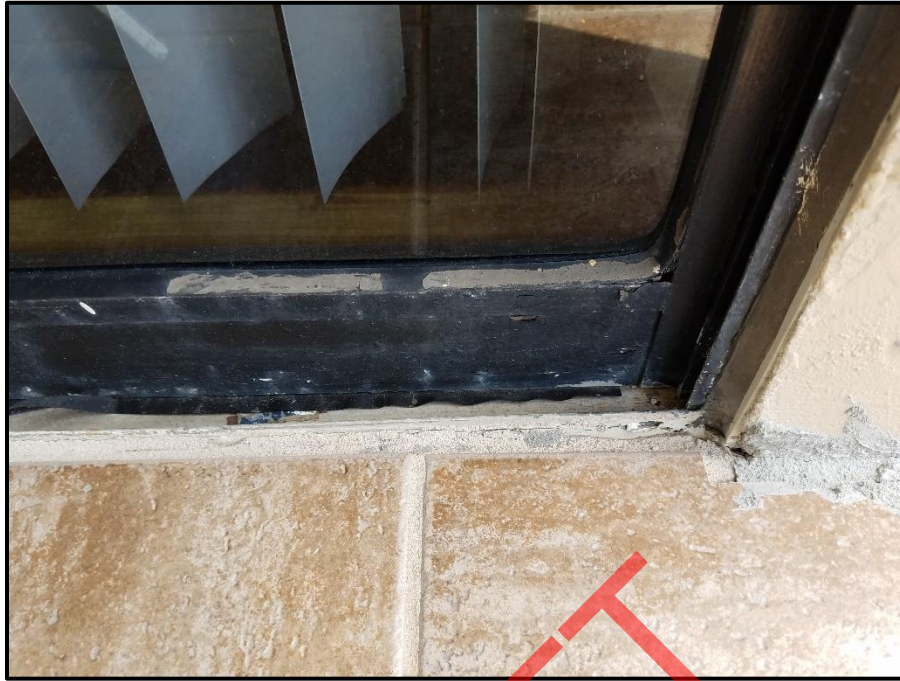
Photograph 31: Unit #402, Void in sealant at bottom right of sliding glass door noted as potential source of water intrusion.
