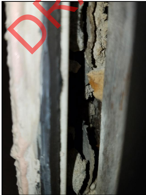
Photograph 26: Unit #204, No sealant at sliding glass door to stucco juncture.
