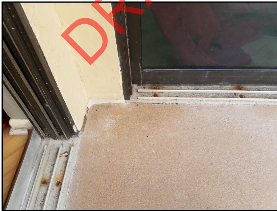
Photograph 70: Unit #301, Corroded fasteners at sliding glass door thresholds observed.
