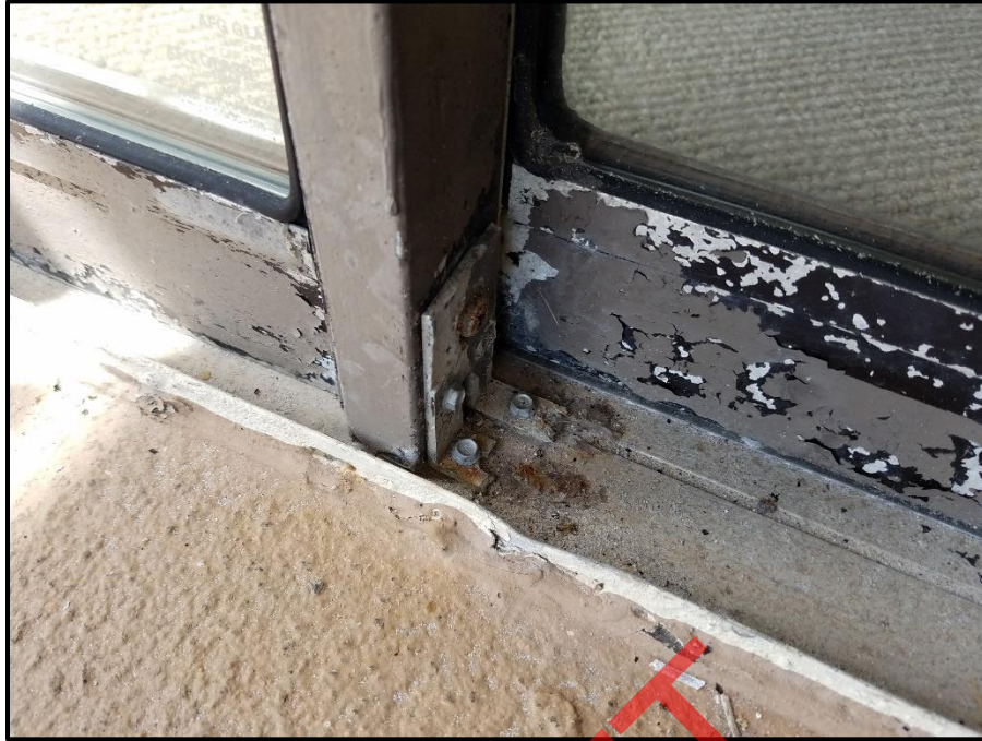
Photograph 37: Unit #403, Sliding glass doors heavily corroded.
