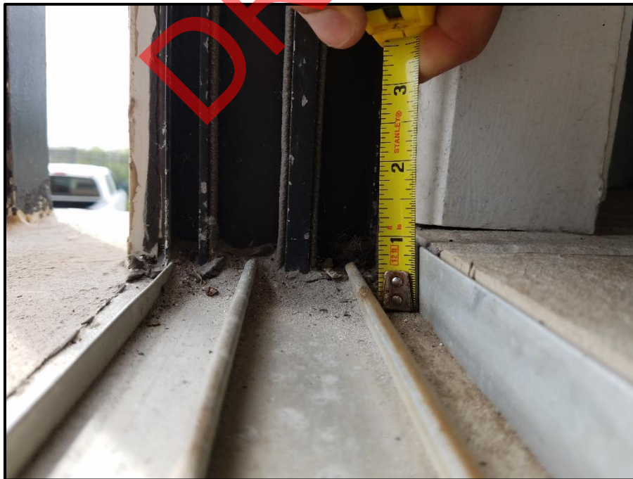
Photograph 12: Unit #203, Rear dam at sliding glass door threshold does not meet code requirement for water infiltration.
