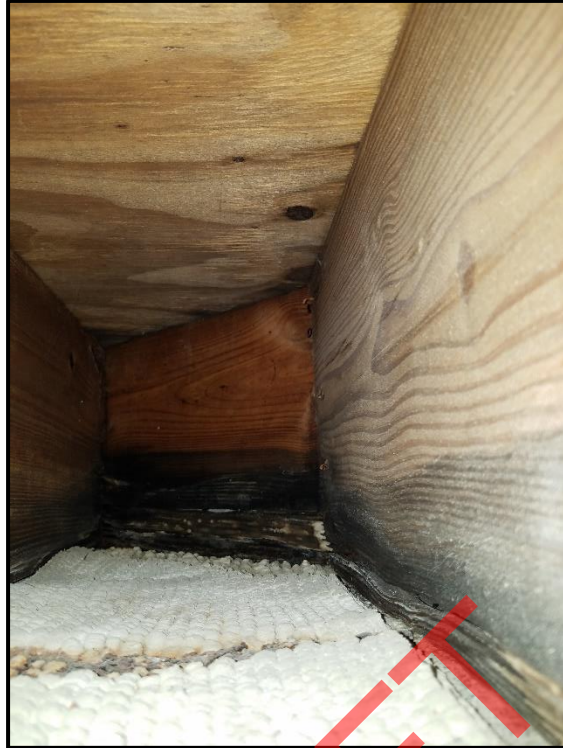
Photograph 3: Unit #203, Bottom edge of floor joists stained and rotting due to water intrusion.
