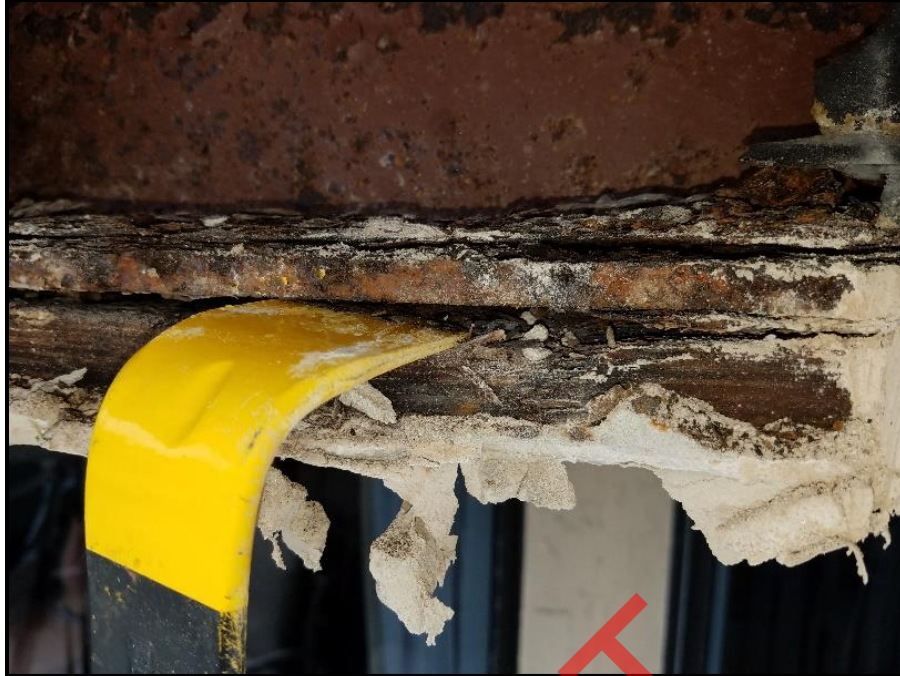
Photograph 7: Unit #203, Wooden buck at I-beam saturated with water and decayed.
