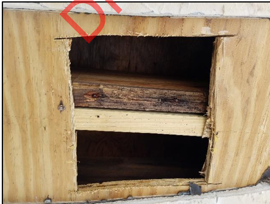
Photograph 18: Unit #204, New joist attached to old joist indicating previous repair attempt.
