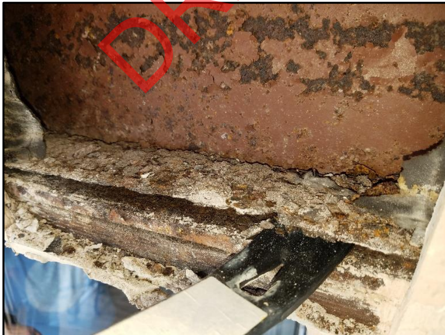
Photograph 6: Unit #203, I-beam delaminating in layers due to long term water intrusion.
