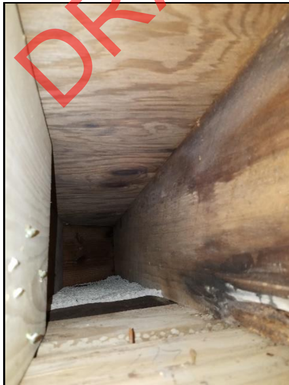
Photograph 20: Unit #204, Interior view of ceiling cavity. Water intrusion. Damaged and/or decayed wood framing.
