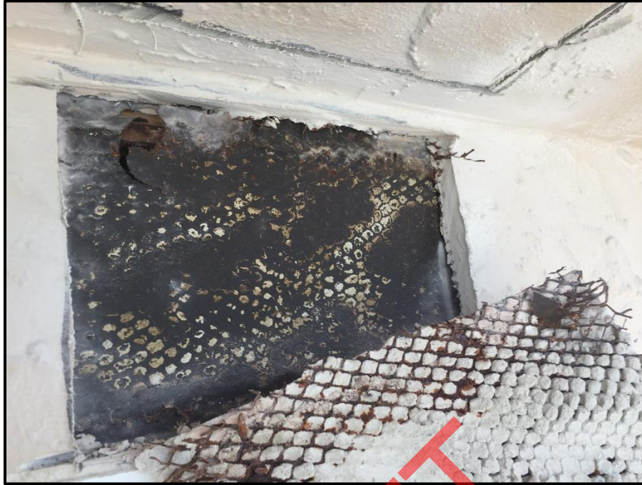
Photograph 89: Unit #304, Observation hole cut at I-beam location, corrosion and staining due to long term water intrusion.
