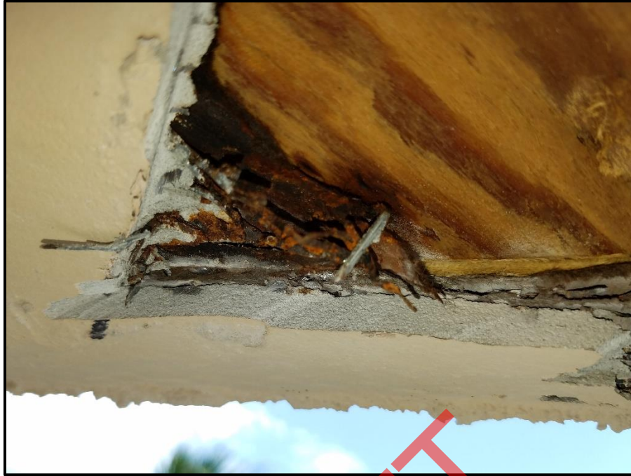
Photograph 55: Unit #202, Heavily corroded stucco lath observed.
