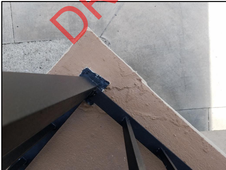
Photograph 86: Unit #304, Crack at leading balcony edge.
