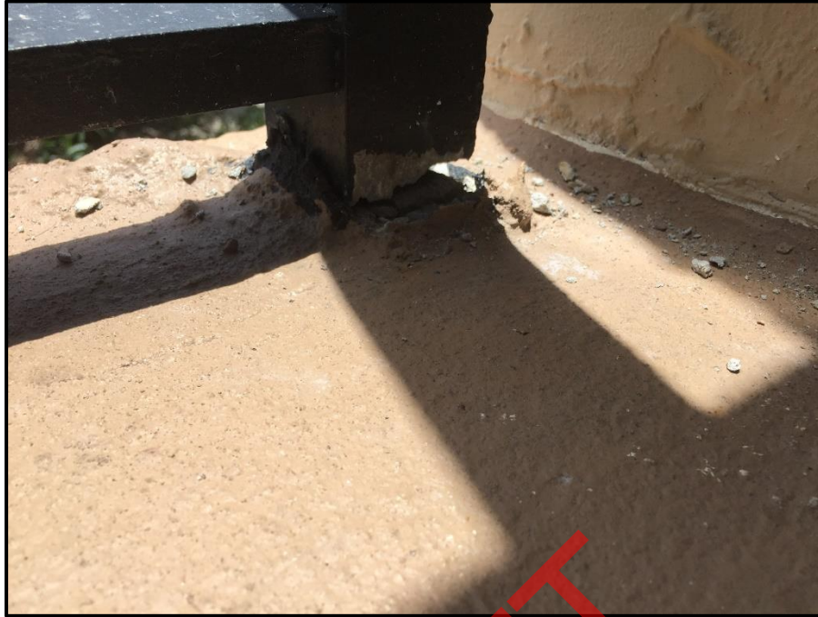
Photograph 59: Unit #202, Guardrail post completely deteriorated due to water intrusion and oxidation.
