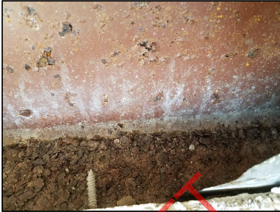
Photograph 75: Unit #303, I-beam corrosion close photo.
