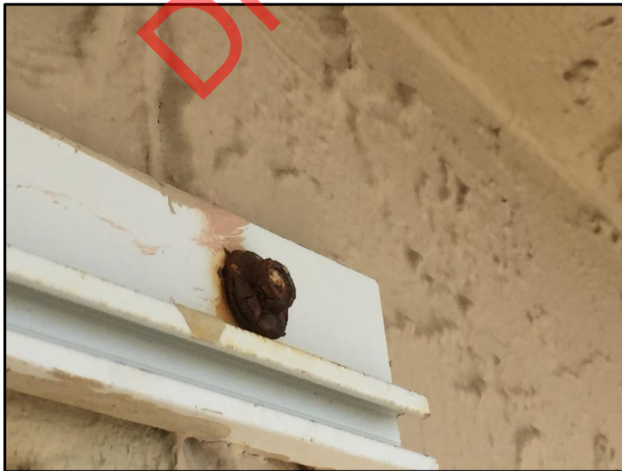
Photograph 50: Unit #404, Heavily corroded fastener at storm shutter bracket.
