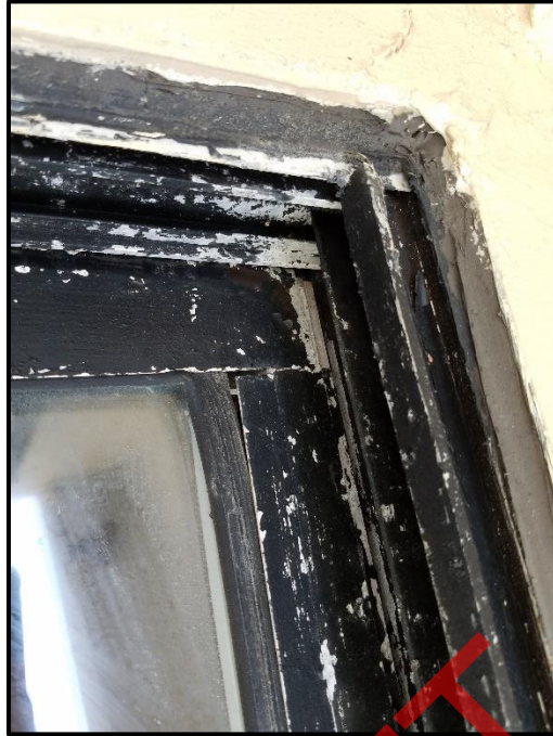
Photograph 77: Unit #303, Sealant failure at sliding glass door.
