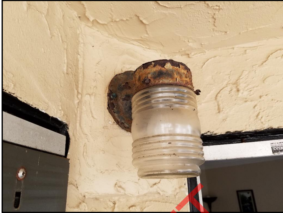
Photograph 43: Unit #401, Balcony light heavily corroded and is not sealed to the wall.
