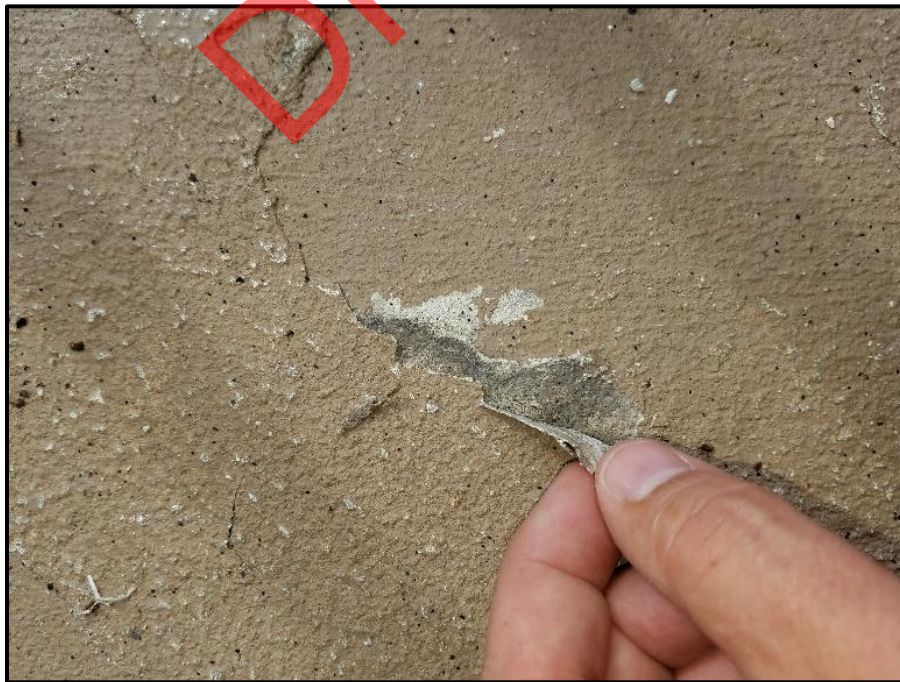
Photograph 14: Unit #203, Water intrusion under acrylic coating.
