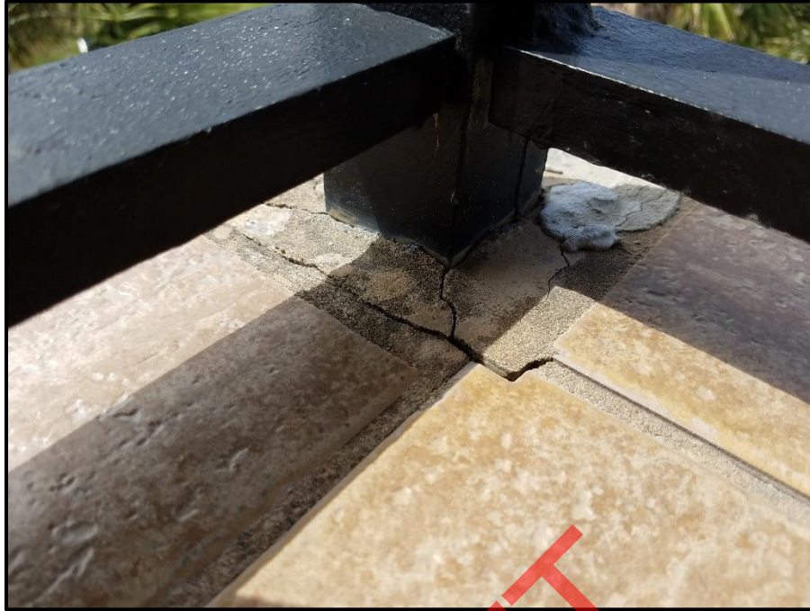
Photograph 29: Unit #402, Grout at guardrail post delaminating due to expansion, contraction and water intrusion.
