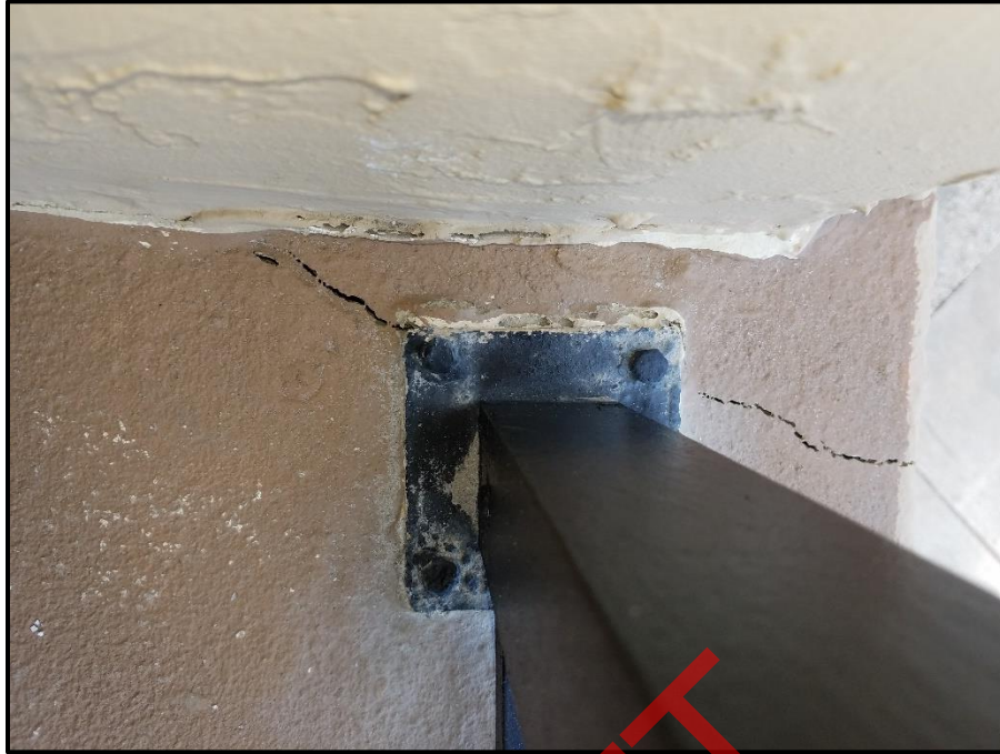
Photograph 85: Unit #304, Crack in topping slab at unit wall.
