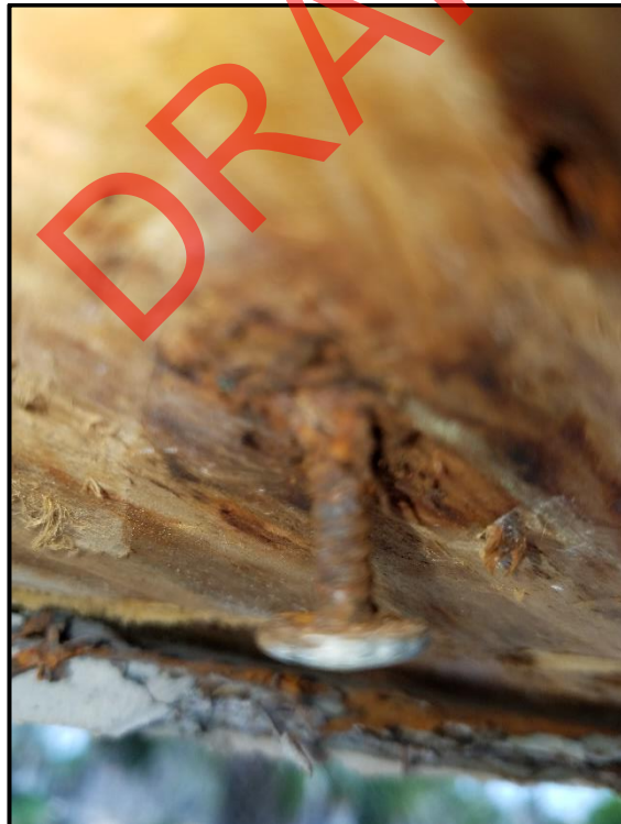
Photograph 56: Unit #202, Heavily corroded fasteners observed.
