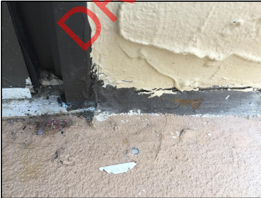
Photograph 62: Unit #202, Sealant failure at unit wall perimeter.
