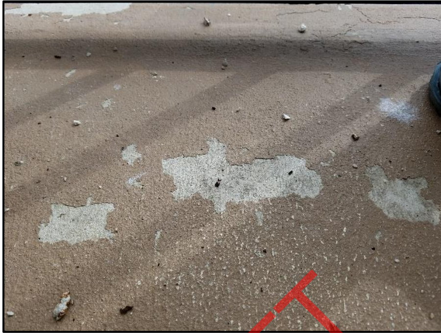
Photograph 13: Unit #203, Acrylic coating on balcony topping slab failing.
