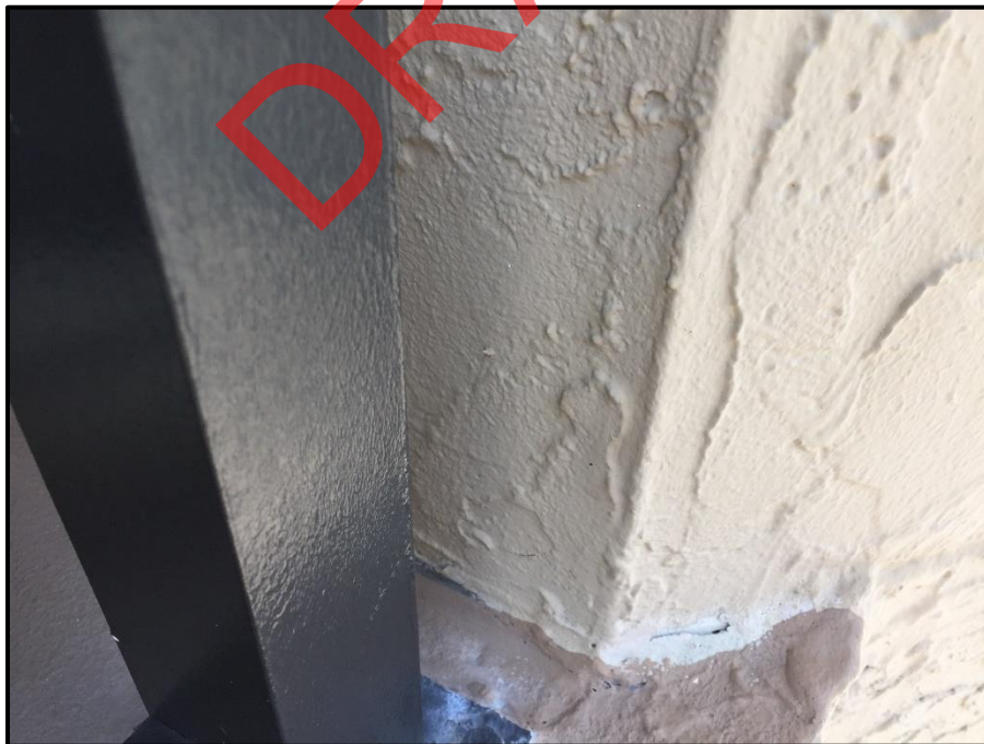
Photograph 44: Unit #401, Sealant failure at unit wall.
