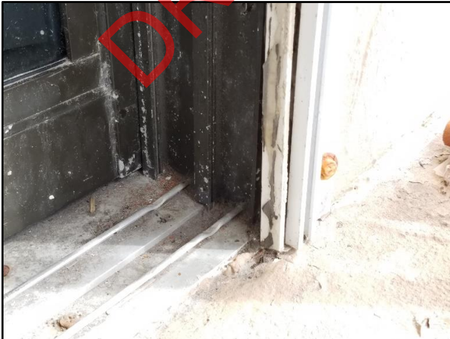
Photograph 24: Unit #204, No sealant at sliding glass door to stucco.
