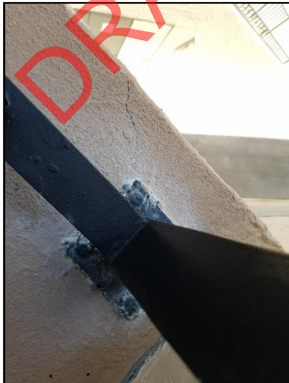
Photograph 42: Unit #401, Leading edge of balcony cracked and spalling at unit wall.
