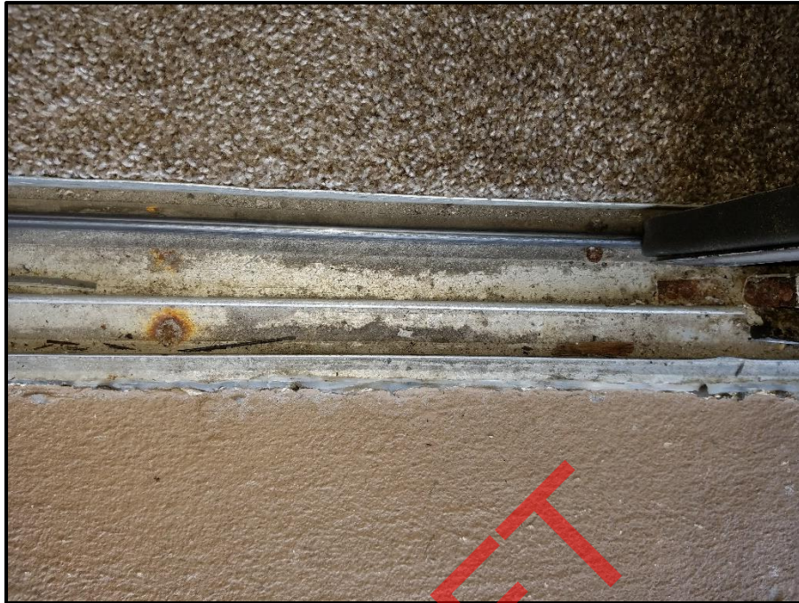
Photograph 87: Unit #304, Rusted fasteners at sliding glass door threshold.
