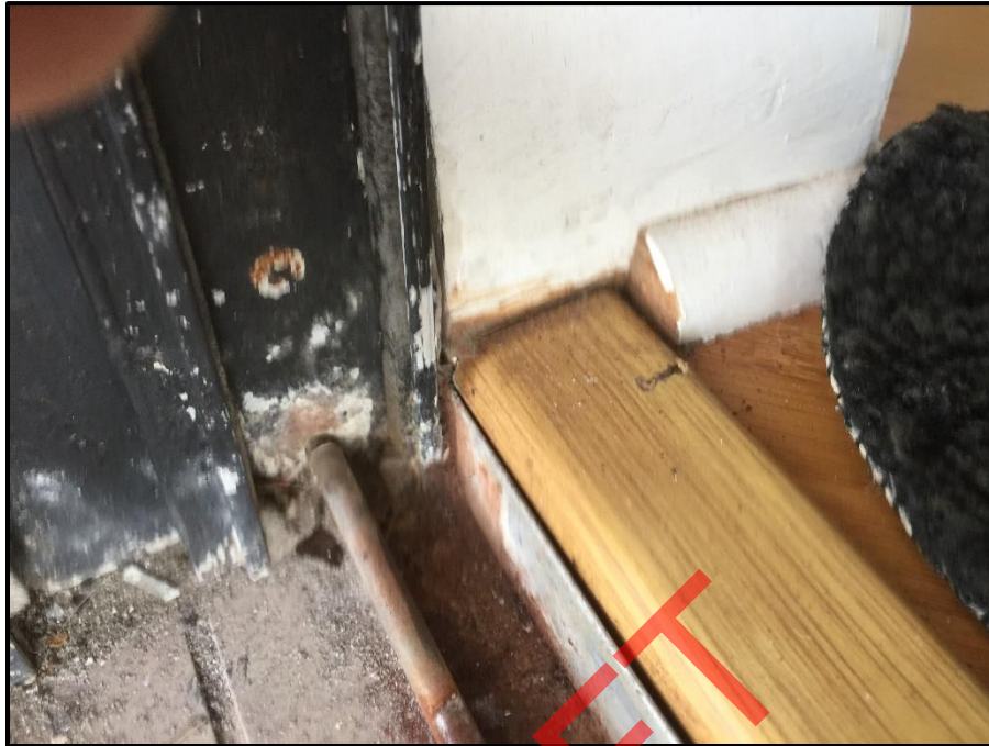
Photograph 33: Unit #402, Evidence of water intrusion noted at rear dam of sliding glass door.
