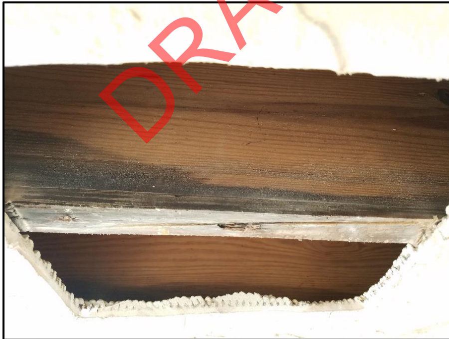
Photograph 2: Unit #203, Bottom edge of floor joist stained and rotting due to water intrusion.
