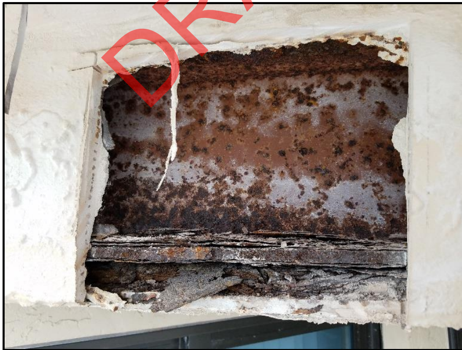
Photograph 22: Unit #204, Observation hole cut in stucco at structural I-beam.
