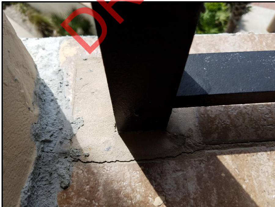
Photograph 30: Unit #402, Grout at guardrail post cracked, allowing water intrusion.
