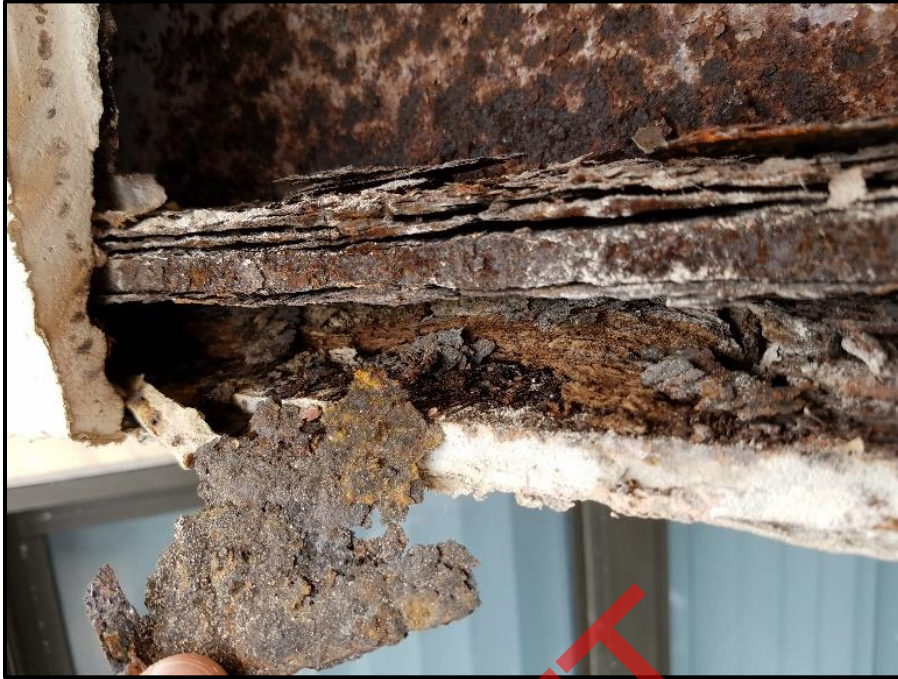
Photograph 23: Unit #204, I-beam and wooden buck heavily deteriorated due to long term water intrusion.
