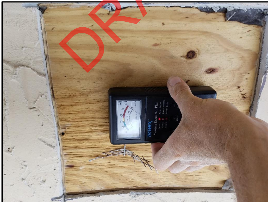
Photograph 66: Unit #301, Observation hole cut in stucco ceiling, high levels of moisture indicated at plywood sheathing.
