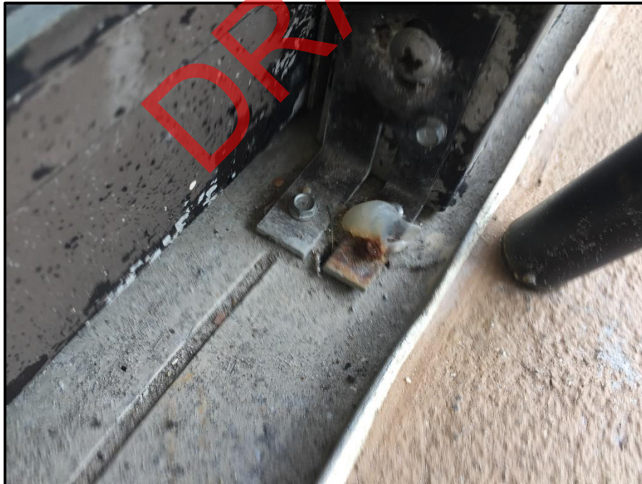
Photograph 38: Unit #403, Sliding glass door fasteners heavily corroded and a potential source of water intrusion.
