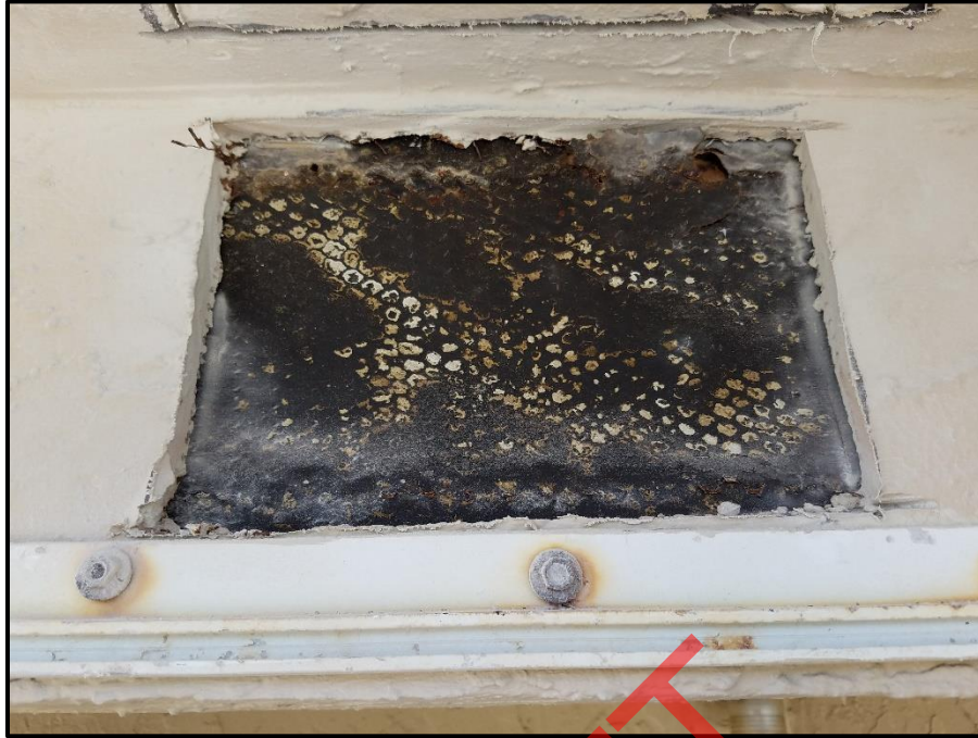
Photograph 73: Unit #303, Observation hole cut in stucco at I-beam location. Felt paper stained due to long term water intrusion.
