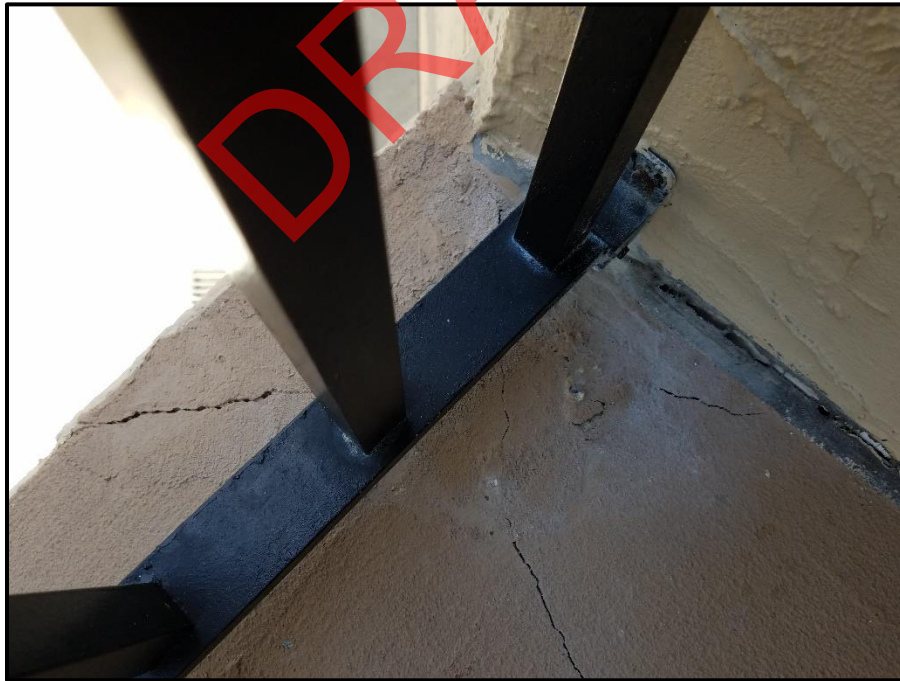
Photograph 64: Unit #301, Balcony topping slab severely cracked at unit wall and leading edge.
