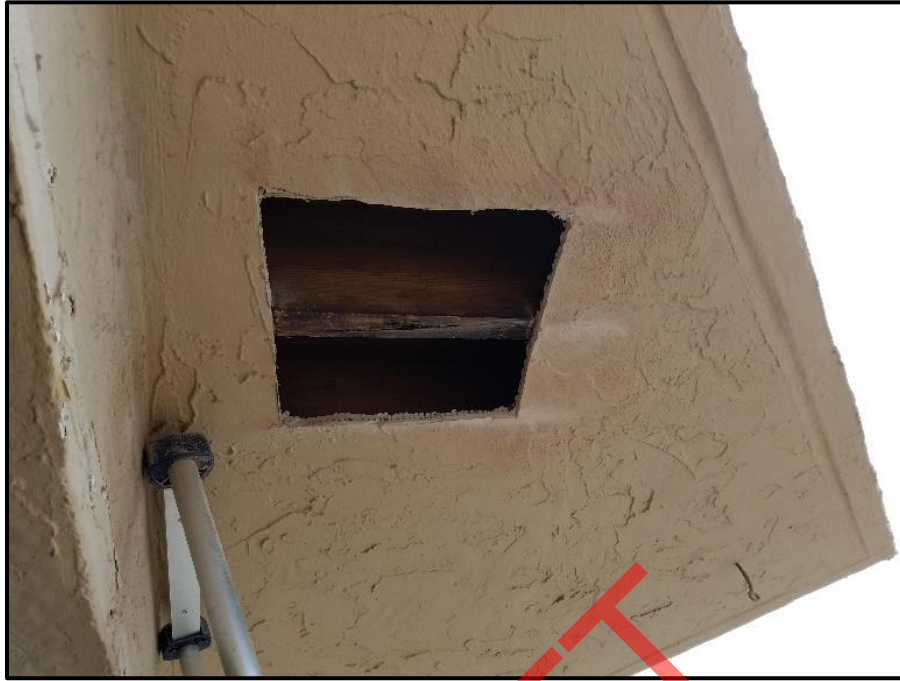
Photograph 1: Unit #203, Observation hole cut in stucco ceiling.
