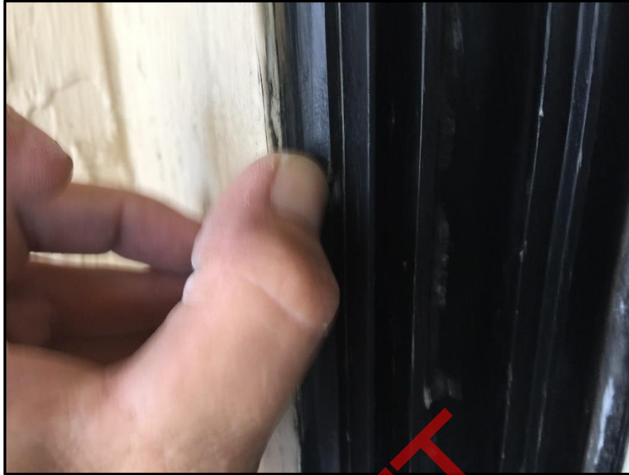
Photograph 45: Unit #401, Failed sealant at sliding glass door.
