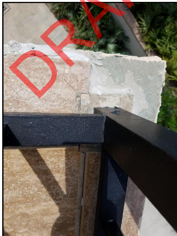
Photograph 28: Unit #402, Leading edge of balcony cracked and beginning to spall.
