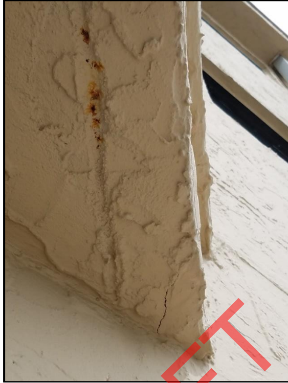
Photograph 21: Unit # 204, Rust stains at balcony edge indicating water intrusion.
