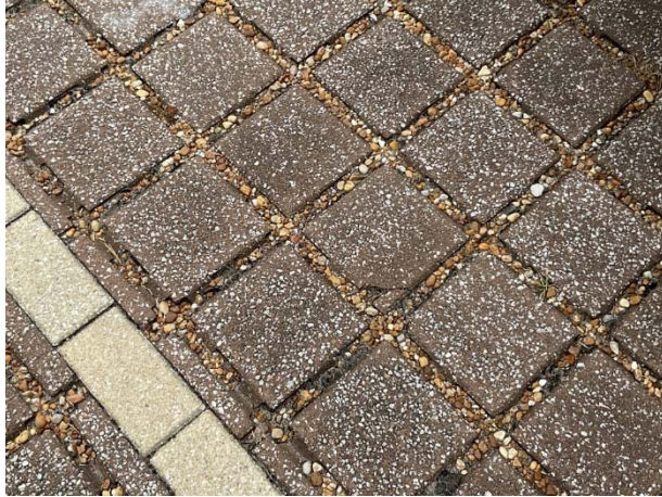
Minor paver damage at parking area
