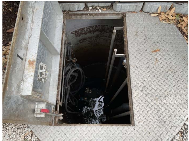
Lift station pit
