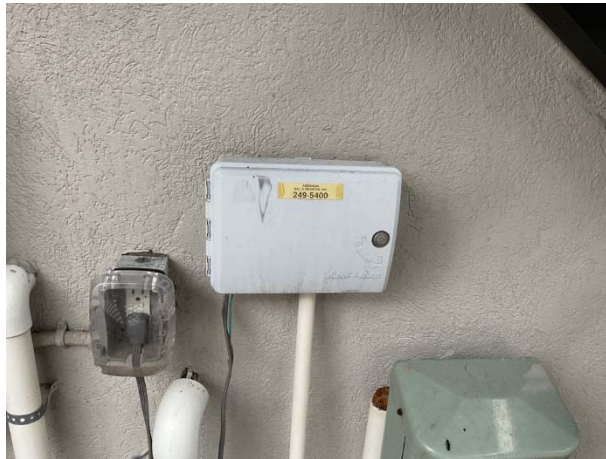
Irrigation system controller
