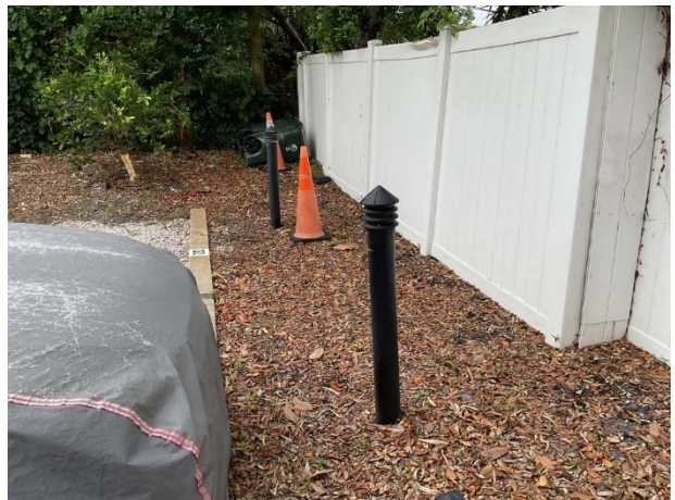
Bollard light fixtures
