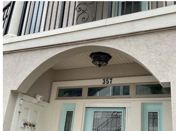
Ceiling mounted light fixture at unit entry
