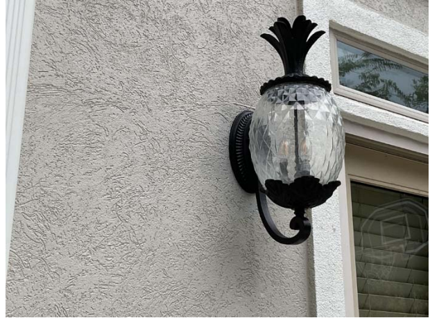
Inconsistent finishes behind light fixture
