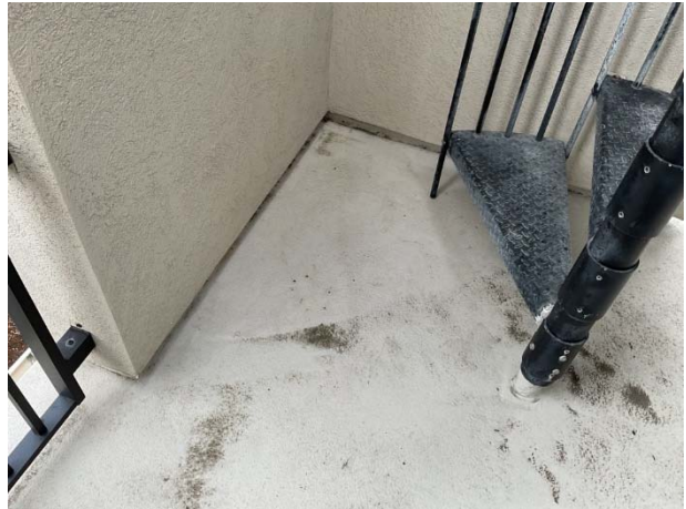
Evidence of standing water
