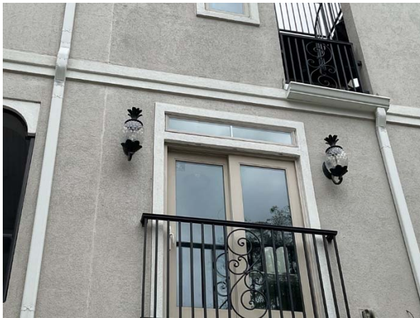
Wall mounted light fixtures
