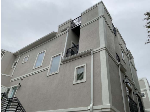
Aluminum gutters and downspouts
