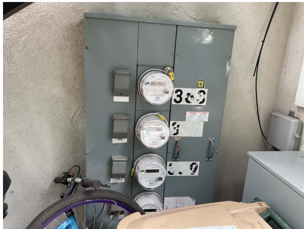
Electrical system main panels
