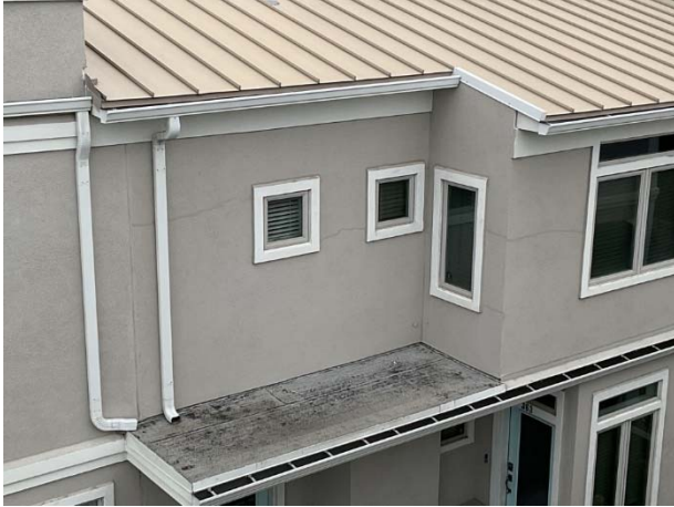
Evidence of previous crack repair
