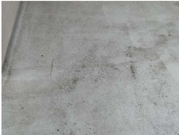
Cracks in rooftop terrace concrete surface
