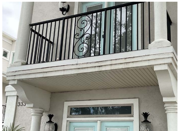
Stucco damage at balcony edge
