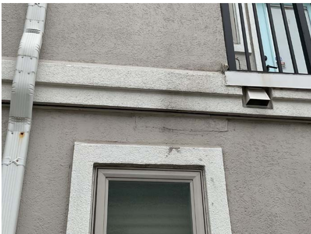
Evidence of previous repair
