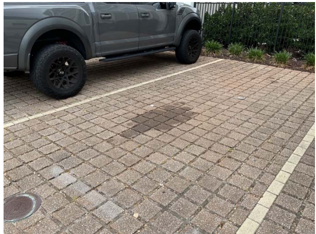
Vehicle fluid stains at parking area
