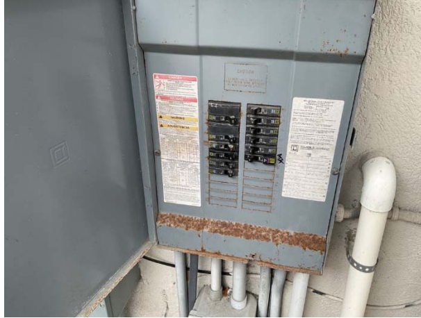
Evidence of water infiltration at common circuit breaker panel
