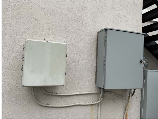
Control panel enclosures
