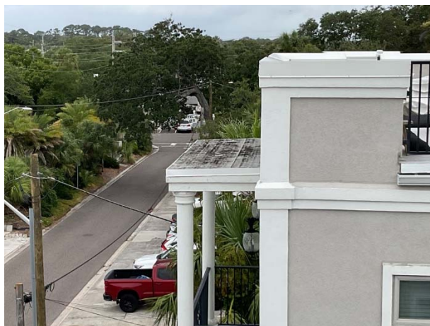
Modified bitumen roof section with evidence of standing water
