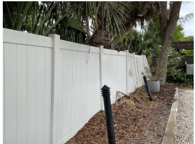
Fence leaning section
