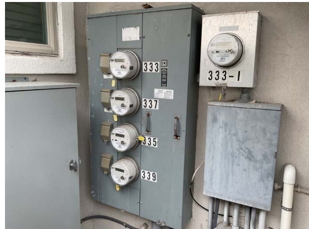
Electrical system main panels
