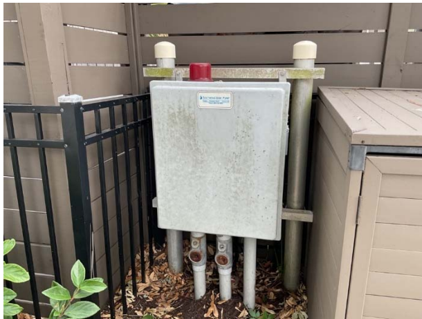
Lift station controls
